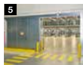
Steel and stainless steel sliding doors
